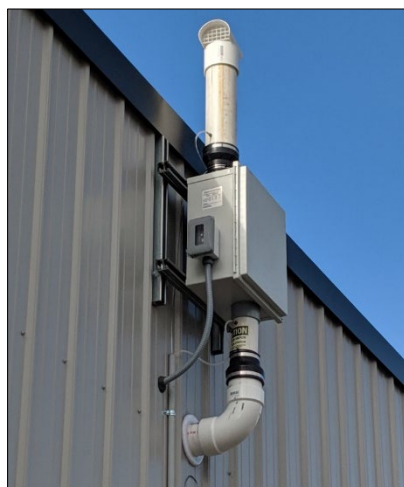
SSD system – outdoor piping and vent stack.
