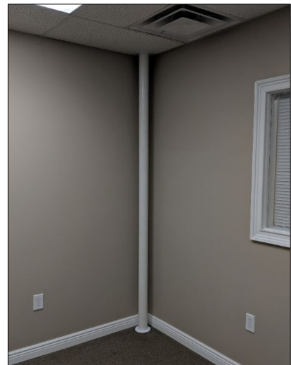
SSD system – indoor piping.
