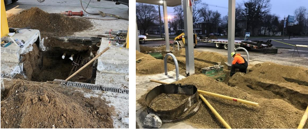
Image (left): Repairs being made to the piping run beneath a dispenser; Image (right): Contractor preparing a site for the installation of new dispensers and piping runs.
